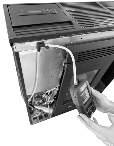
Fig. 46 - Digital pressure switch connection
